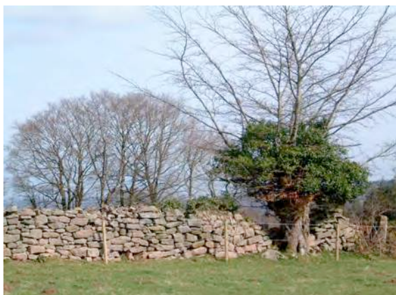
Wall damage caused by a tree
